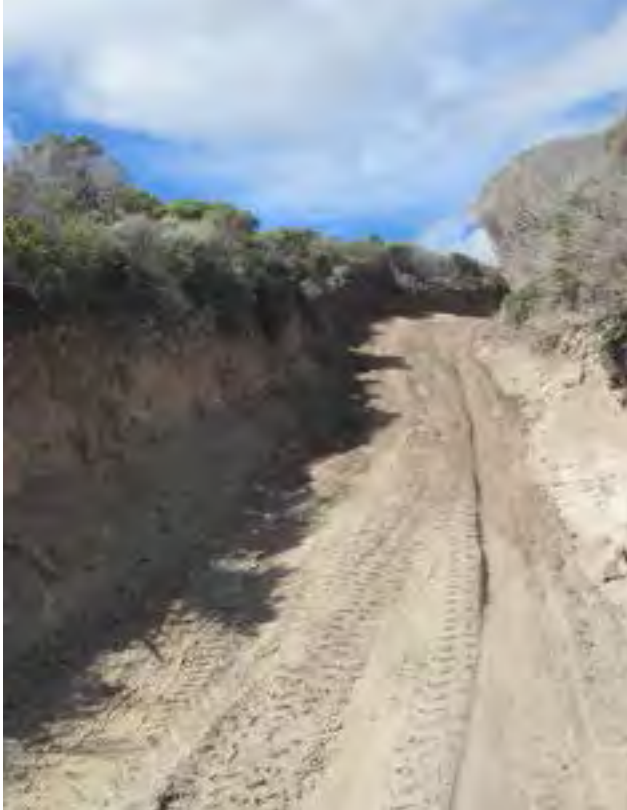
Erosion on vehicle access tracks to the coast pose an ongoing management concern. Photo – Parks and Wildlife
